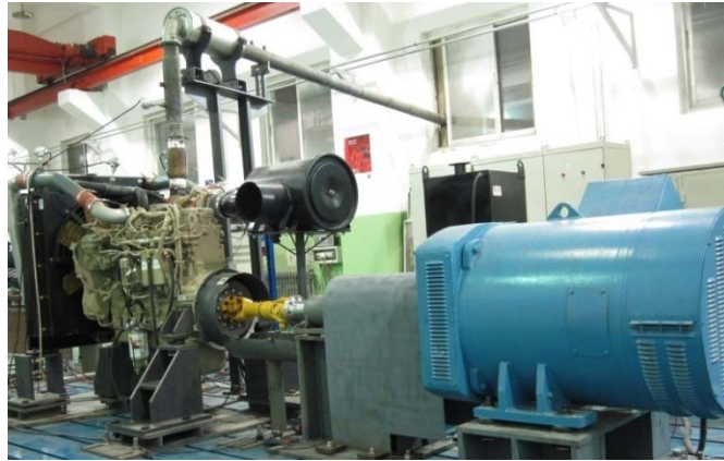
Figure 2. Diesel electric group and generators
