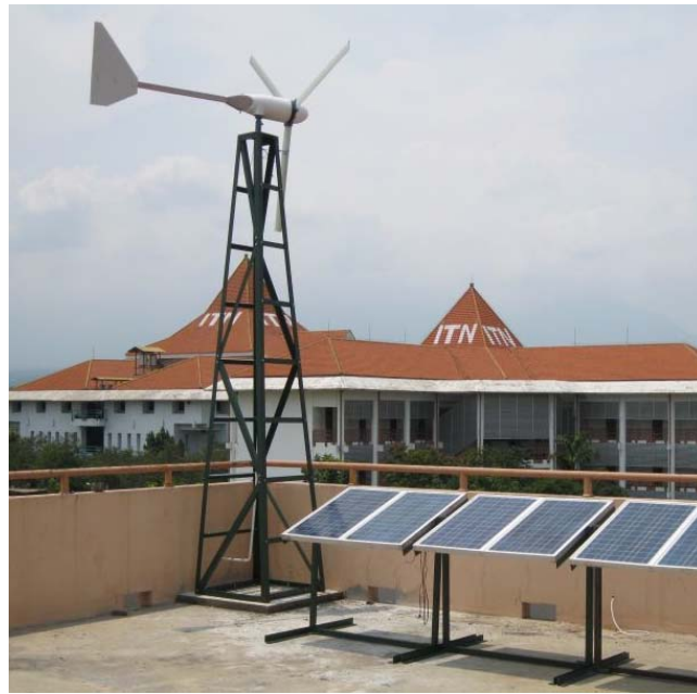
Figure 3. Wind-PV power system.
