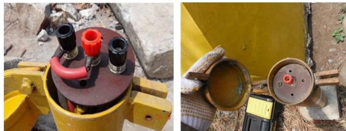
Figure 5. Measurement point of cathodic protection system
