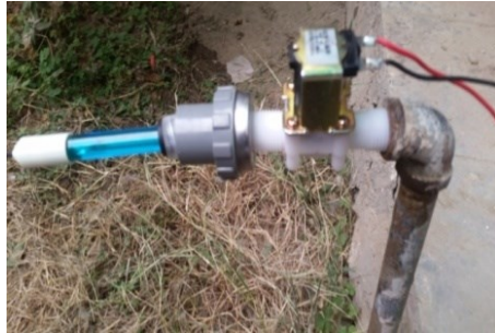
Figure 7. Solenoid valve connecting to tap water pipe
