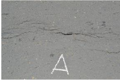
Figure 2. Road surface cracking image
