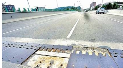
Figure 3. Failure of the comb-plate expansion joint in Tang-Min Bridge, China in which the right plate popped up because of the failure of the anchor bolts
