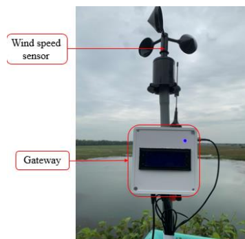
Figure 9. In the experimental area, the gateway circuit is equipped with a wind speed sensor
