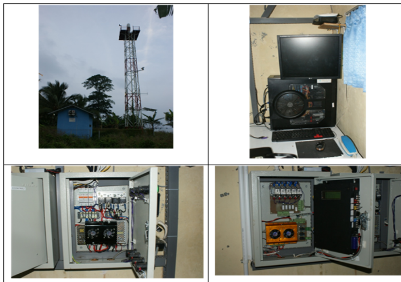
Figure 6. Merak Radar Station
