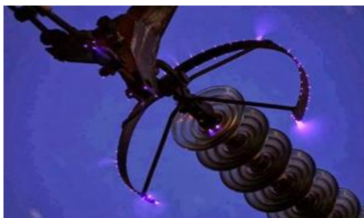
Figure 3. Corona discharge on an insulator string of a 500 kV overhead power line [4]
